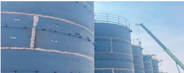
Green Hydrogen-Ammonia-Alcohol Integration EPC Project - Demineralized Water Preparation System Equipment
