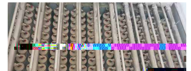
Rongcheng Water Plant, Xiong'an
