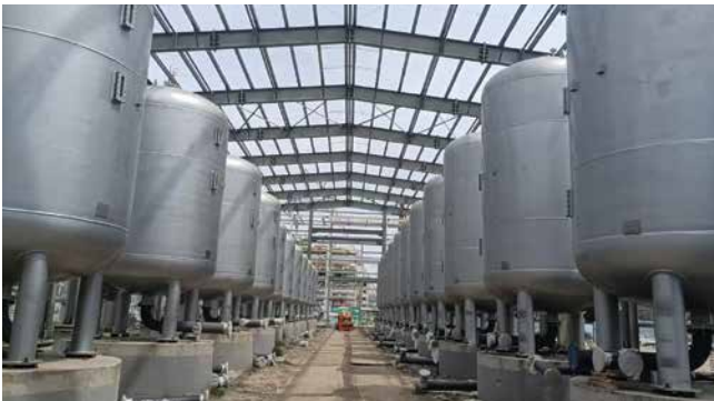
North Huajin United Petrochemical Co., Ltd. Fine Chemicals and Raw Materials Project - Condensate Water Station Complete Equipment Capacity:2500t/h+750t/h Process:Utility Engineering Area: Primary Filter+Secondary Filter+Activated Carbon Filter+Prepositive Cation Bed+Mixed Bed Refining Area: Primary Filter+Secondary Filter+Activated Carbon Composite Filter+Prepositive Cation Bed+Mixed Bed
